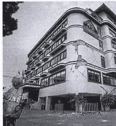
This hotel facade shows damage from the 6.3-magnitude quake.
