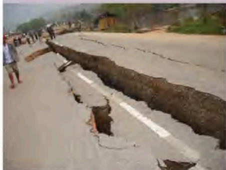
Roads were damaged during the March 24 earthquake
